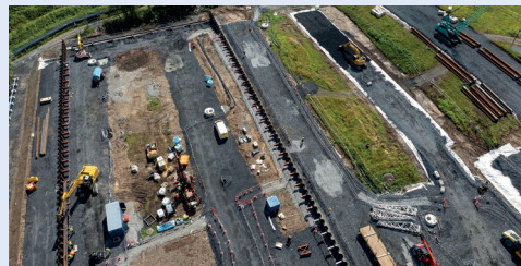
August 2024: Sheet piling in place to enable the construction of the first enclosure on the landfill.
