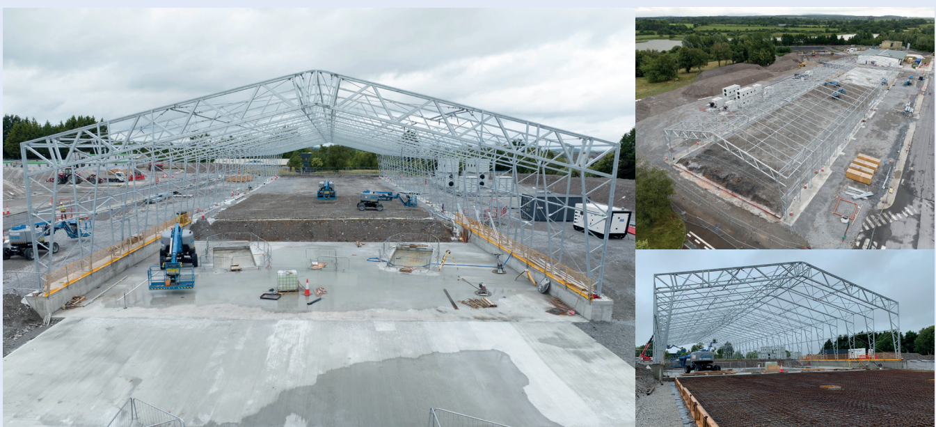
Stage 2: The building of the steel frame that will support the enclosure cover.
