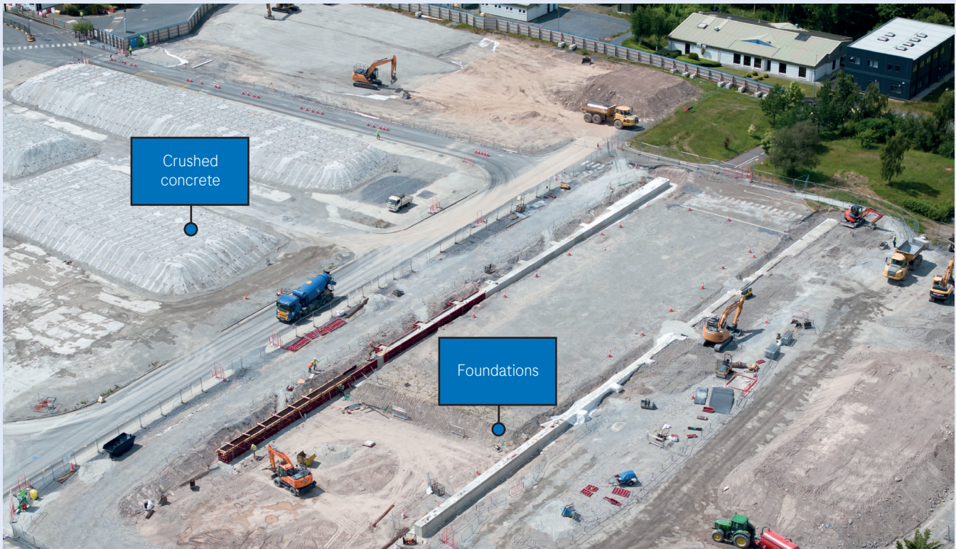
Stage 1: The preparation of the ground and the foundations. The enclosures have been designed to operate under high wind conditions and this has been reflected in the specification of the foundations installed.
